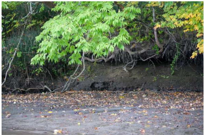
2024 CRC Site 9 (21) Close-up of eroded area
