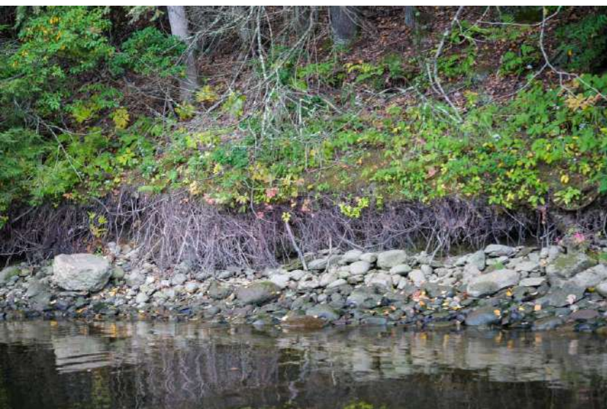
2024 CRC Site 1 (18) Exposed roots above water fluctuation zone
