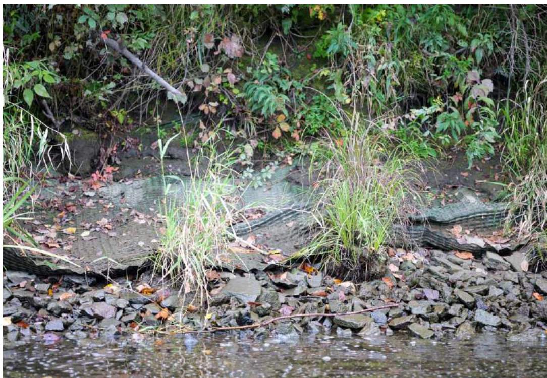
2024 CRC Site 12 (7): Previous restoration site with unsightly material trying to hold the riverbank together
